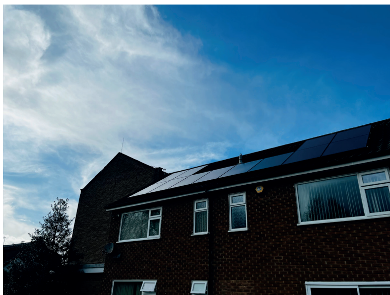
Solar panels installed last year at St Clare's Presbytery in Acklam, Middlesbrough
